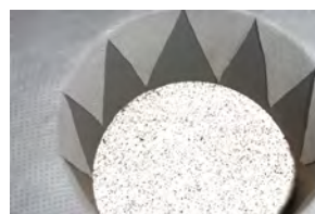
Paste the sheet neatly into the walls of the sump, and with it ....
