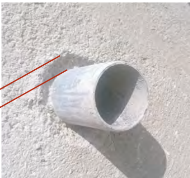
Open the area around the pipe in a "V" shape. THIS WIDTH IS INSUFFICIENT!!
