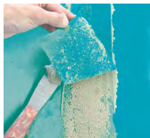
Apply EPOXICOL between the sheets of LAMINAS to attach the BANDA-SOLAPES waterproofing strips.
