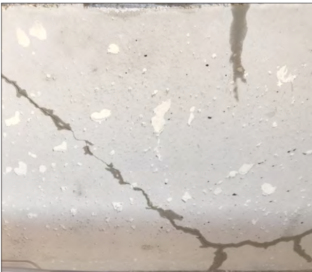
Concrete with micro-cracks that cause leaks in a pool or tank.
