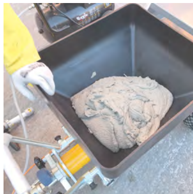
Next, pour the mortar already mixed with the water in the hopper of the projecting machine and ...
