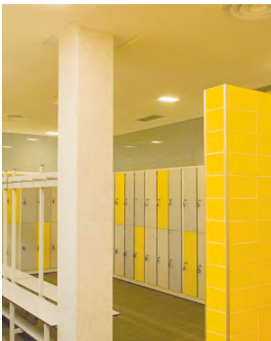
Grouting of mosaic and ceramic tiles in areas subject to intense physical-mechanical wear.
