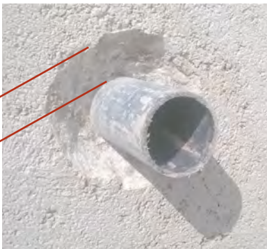
This WIDTH and this DEPTH are correct.
